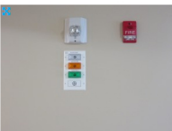
Each apartment features lights and other equipment to let residents know if there is an emergency or someone is at the door.
