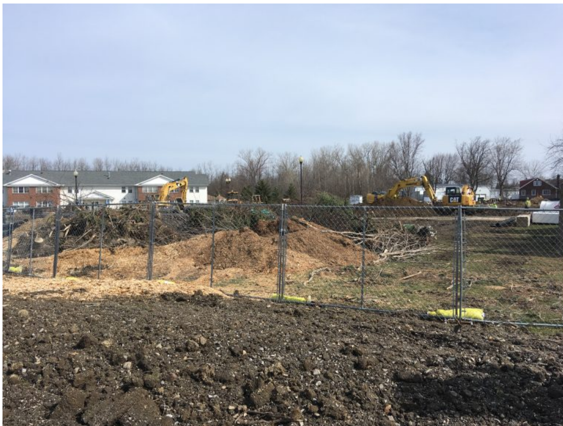
Workers prepare the land for the Apple Blossom Apartment complex on Old Union Road. (Jim Herr/Cheektowaga Chronicle)
